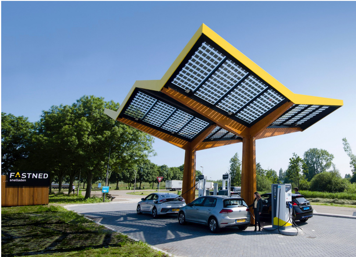
Fastned De Watering, our first station with 175 kW (and 350 kW ready) fast chargers.
